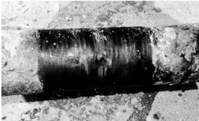
Picture 1: big leak
