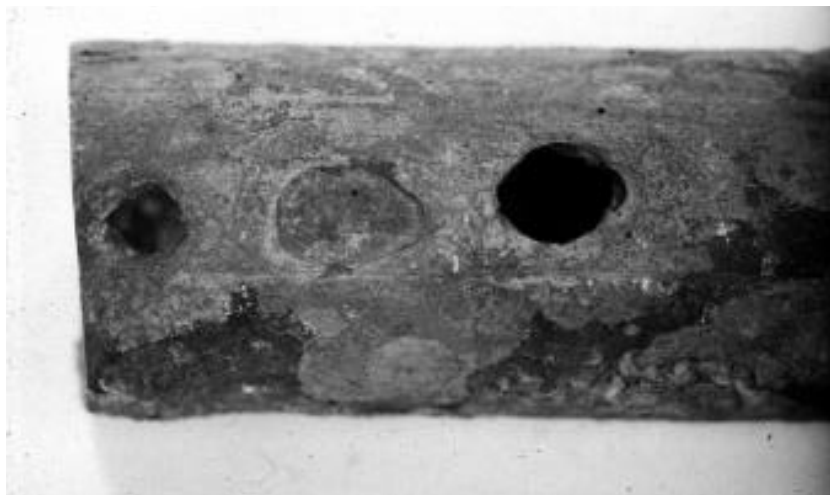
Picture 2: leaks caused by corrosion from the outside
