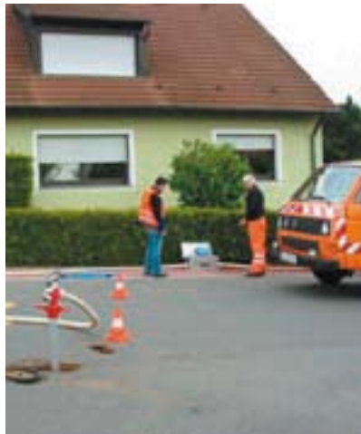
Picture 12: Zero Consumption Measurement – Installation
