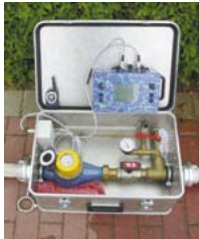
Picture 13: Zero Consumption Measurement, measuring of flow and pressure
